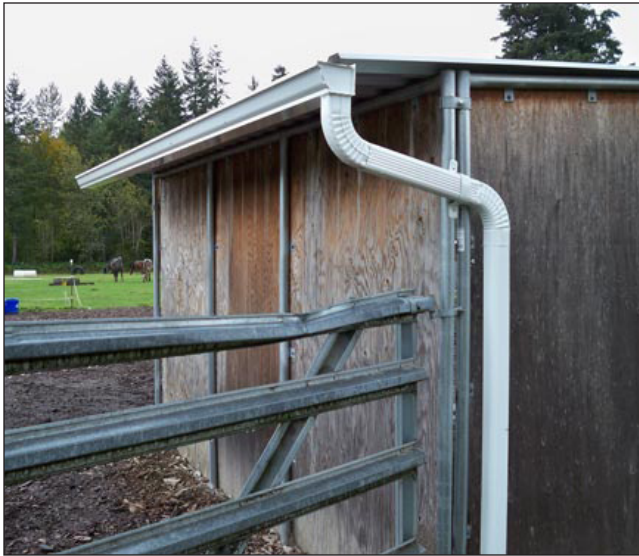
Figure 25. A roof runoff structure like the one pictured helps collect, control, and transport precipitation from roofs. Photo courtesy of the King Conservation District.
