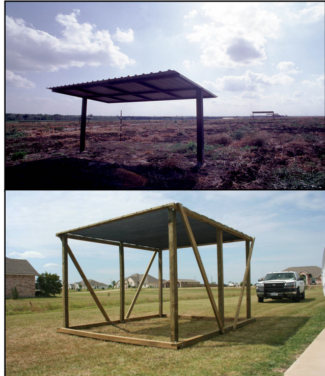
Figure 14. Shade structures constructed with a tin roof (top) and a shade cloth (bottom). Photos courtesy of The Samuel Roberts Nobel Foundation Inc. (top) and Larry Redmon, Texas AgriLife Extension Service.
