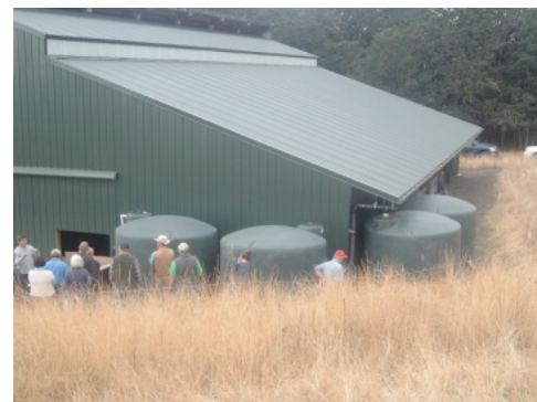
These four 2,500 gallon water harvesting tanks capture rainwater from the barn's roof and help save over 162,000 gallons of water a year that would otherwise be pumped from the groundwater aquifer below. Photo courtesy of Yamhill Soil & Water Conservation District.
